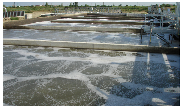
Nitrification unit using dish aerators.
