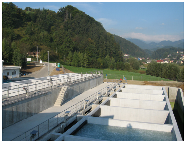
Post-Treatment by Biological Activated Filtration and subsequent Denitrification Filtration
